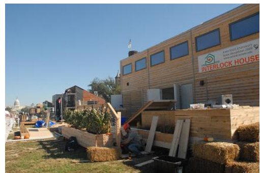
The Iowa State team's entry included the use of soy-based spray foam insulation.
